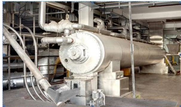
Figure 3 Drier of incineration plant
