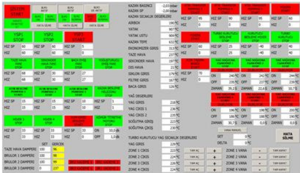
Figure 10 Operator panel for entering operation values
